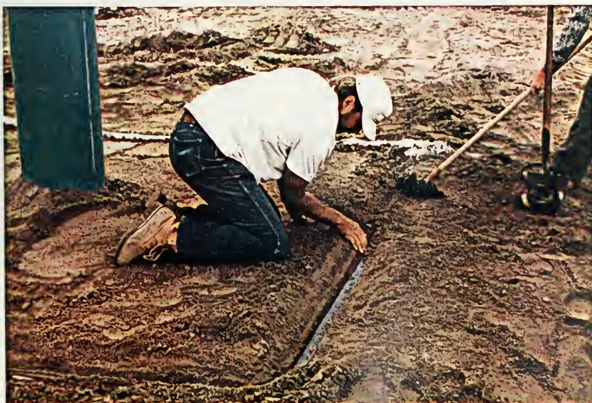
A20: BENTONITE SEAL PLACED ALONG TOP OF LINER TO PREVENT PREFERENTIAL FLOW ALONG LINER WALL
